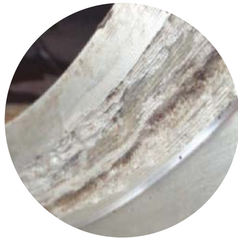
An example of corrosion caused by use of conventional graphite gaskets.
